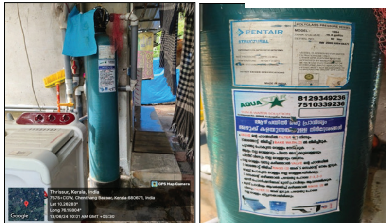
Figure. 29: Some of the filter point wells used by residents of SN Puram
