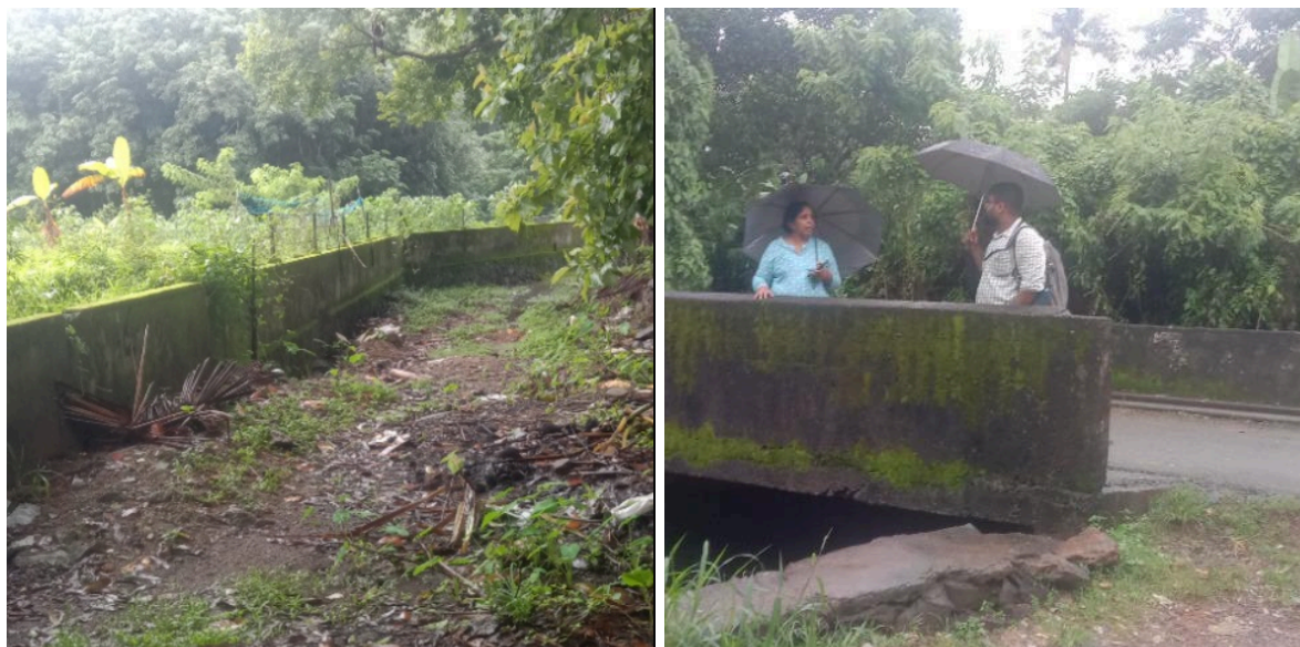
Figure 32: Blocked drain due to compound wall and bridge
